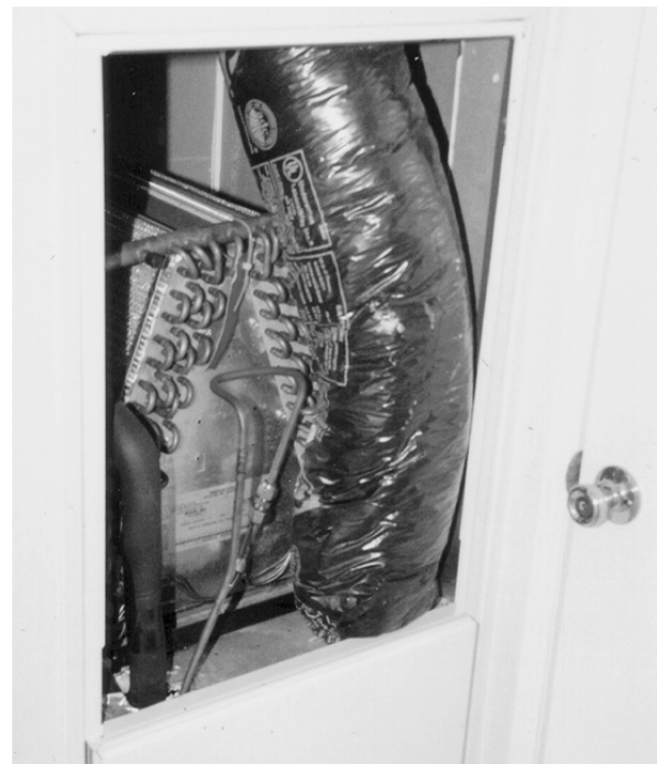
A correctly completed installaton: furnace with aftermarket air conditioner.
