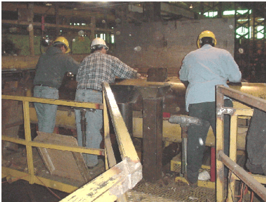
Elevated work platform and catwalk in front of conveyor
